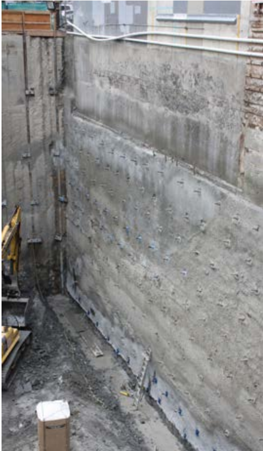
Fig. 2: 41 ft (12.5 m) deep shotcrete underpinning below the bottom of an existing building footing on the east elevation
