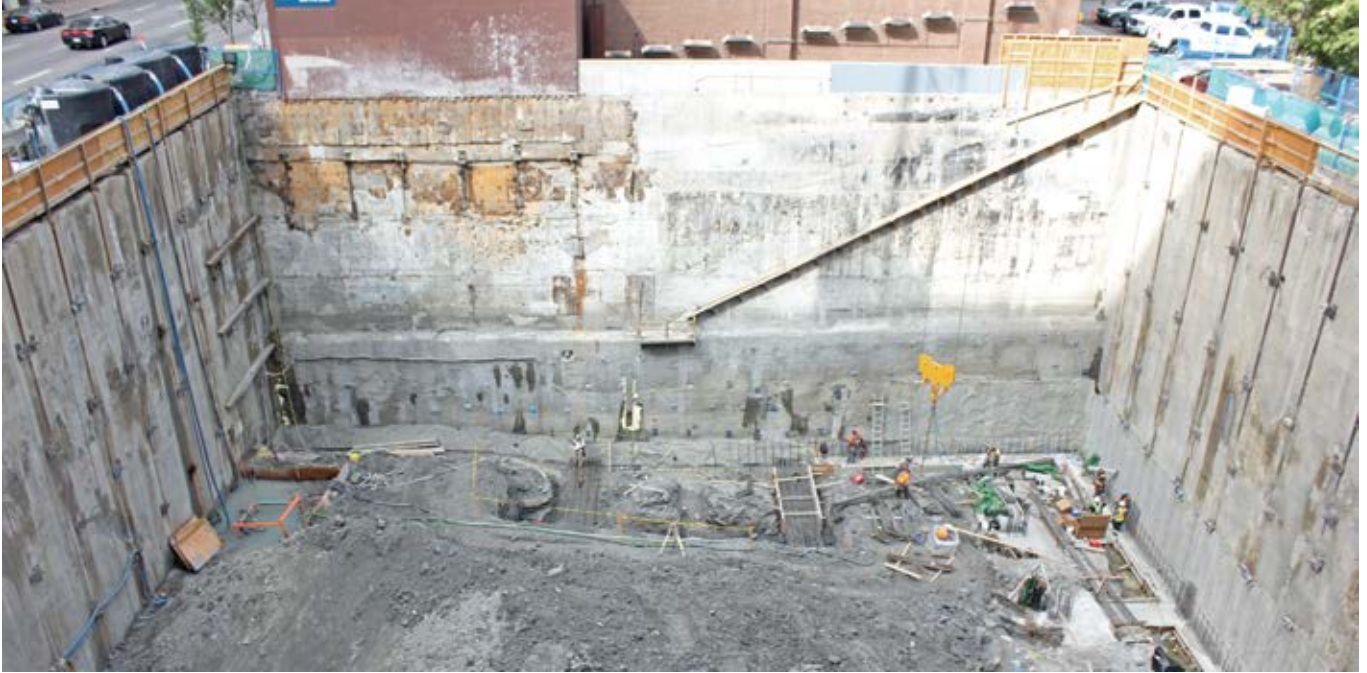
Fig. 1: 21.3 ft (6.5 m) deep shotcrete underpinning below an existing building footing on the west elevation at The Vogue, Calgary, AB, Canada
